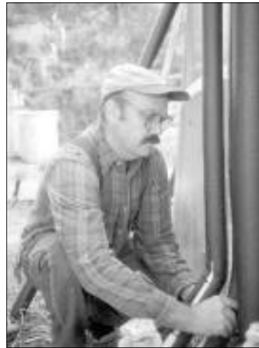
David Nelson from Esalen's Maintenance Crew works on the pipe insulation for the 1,500 gallon holding tank at Porter's Yurt.
