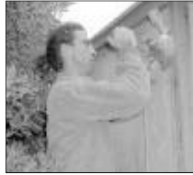
Peter Littlejohn , an Esalen Staff member on the Maintenance Crew, works to finalize the electrical system for the new redwood tubs.
